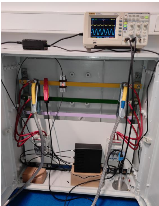
Fig. 3a. Photo of the switching box with installed one OFCS-EC sensor.
